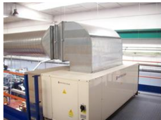
Heat pump building 2
